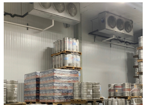
Motor upgrades to evaporator fans help control energy usage in keg cooler spaces at the Mockler facility.
